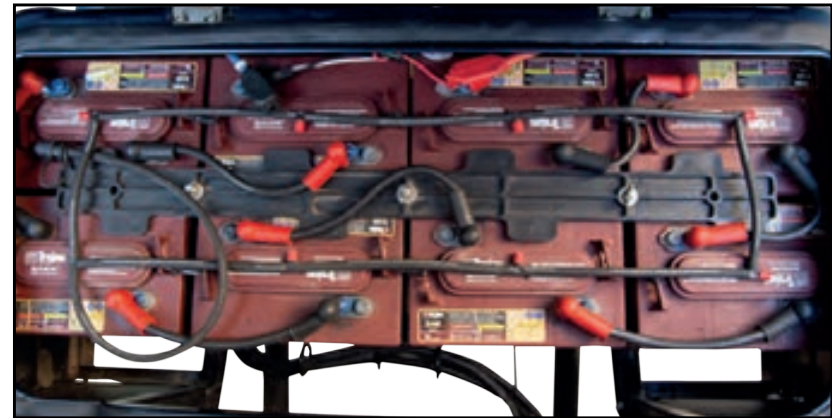
Automatic Battery Watering System
